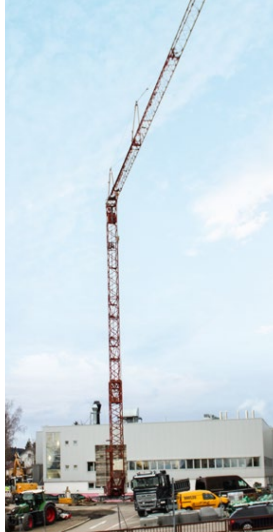
With the help of a Liebherr crane, construction site activities are progressing quickly.
